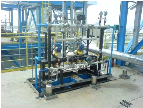
Skid made of plastics for SCR in one incineration plant ( \text{NH}_3 injection)
