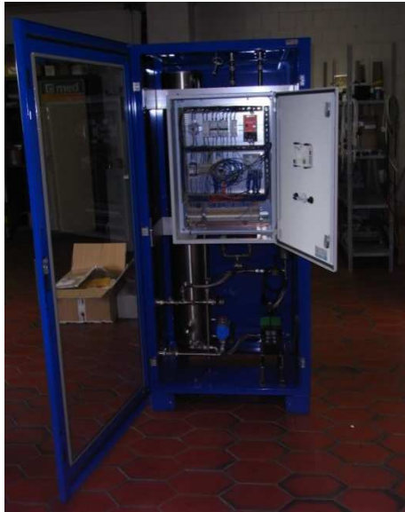
Urea dosing rack for diesel generators
